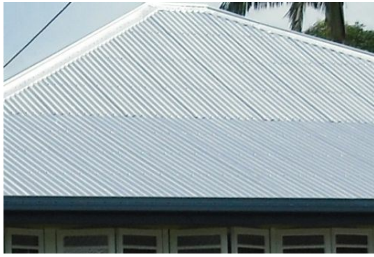
Figure SC6.2.3.22 Corrugated galvanised iron is typical for roofing in Townsville Character buildings
